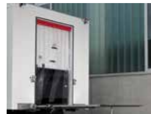
Rear rolling shutter gate
